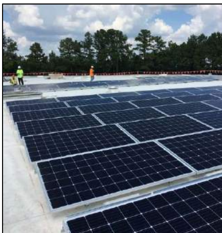
FODAC's 100 kW system is atop its warehouse in Stone Mountain, Georgia.
