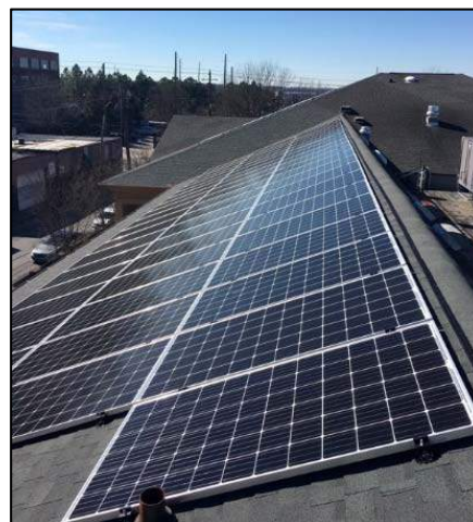
Red Shield Shelter's 28 kW system.
