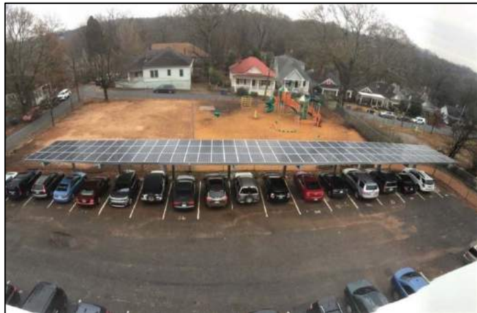
ANCS's 41 kW solar carport canopy is projected to save the school over $6,000 a year.
